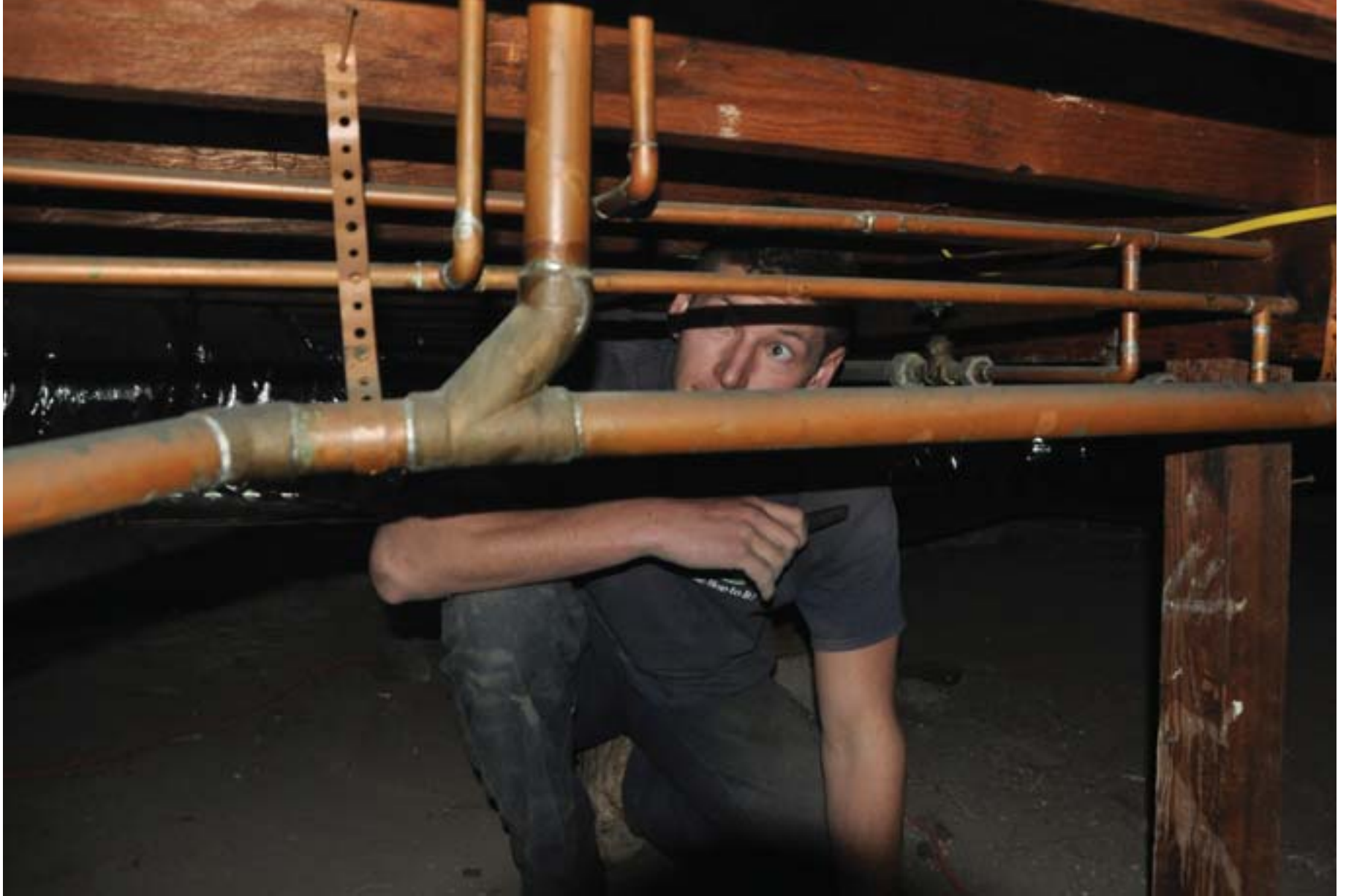
Leapfrog Plumbing technician Austin Barber inspects the newly installed copper pipes under a house.
